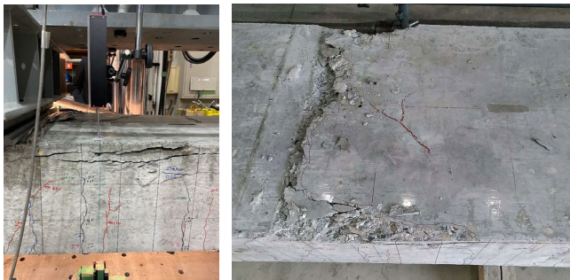
(a)Side (b)Top surface Fig.9 Crushing of concrete
