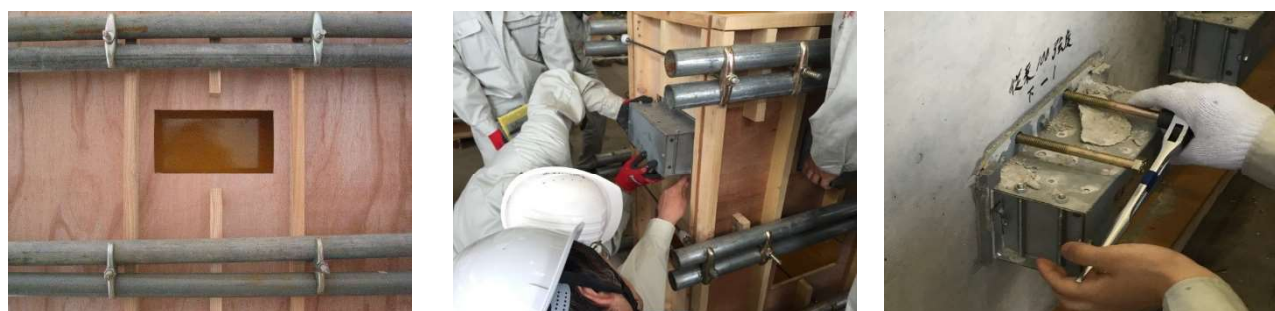
(1) Hole in sheathing board
